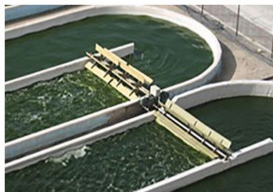
Photo 4-Algal Turf Scrubber (ATS) system
