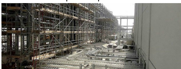
Figure 3 – Sadara Power and Piperack Interface (3)
