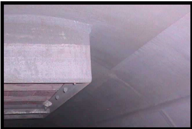
Picture of water mark on the steam drum
