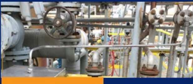
▲ The picture is a home made system and consists of a pipe from the process line to a sulfuric acid sample box. The pipe from the valve (top right) to the sample box (bottom left) must be purged before a representative sample can be taken. This not only produces waste, but if not flushed correctly leftover residue may influence the next sample.
