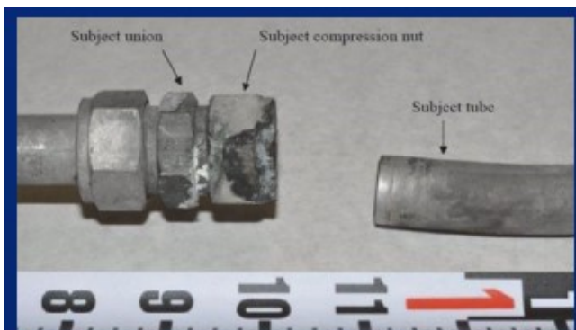
▲ A loose section of tubing connection from a sulfuric acid sample station responsible for the release of 84,000 pounds of sulfuric acid into the environment. 4
