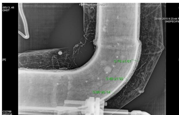
Figure 10 : CR Radiograph Showing Corrosion Deposits.
